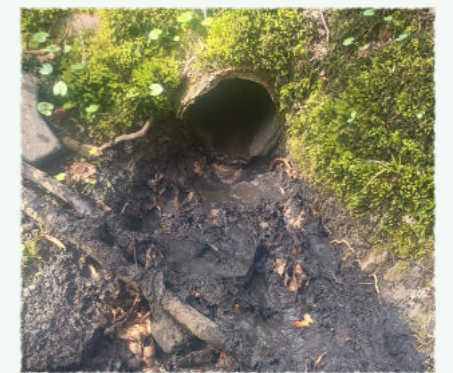
Figure 6, A surface water outfall on Gledhow Valley Road discharges directly into Gledhow Beck. Black sludge flowing from the pipe is the result of Leeds City Council's road gully cleaning.
