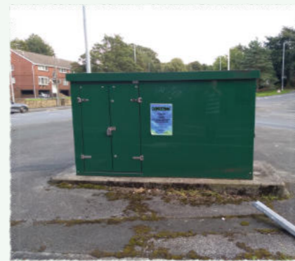
(1) Harrogate Road CSO-above ground control cabinet
